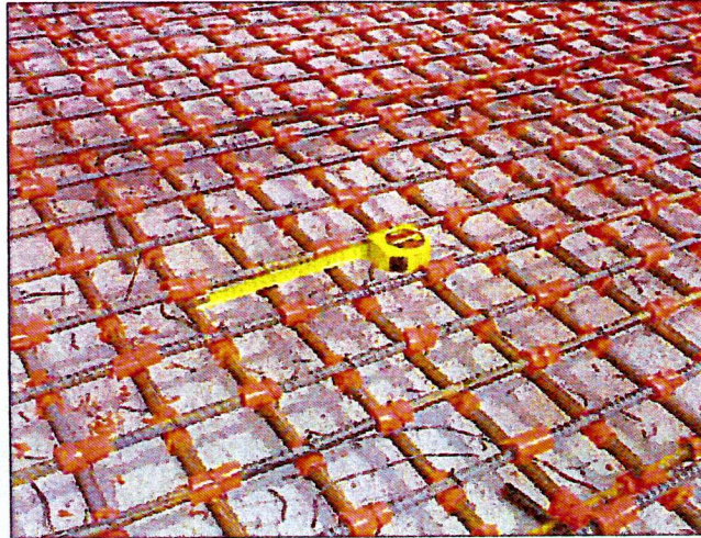
Picture 14 – Magnetic insulation of the ground grid
